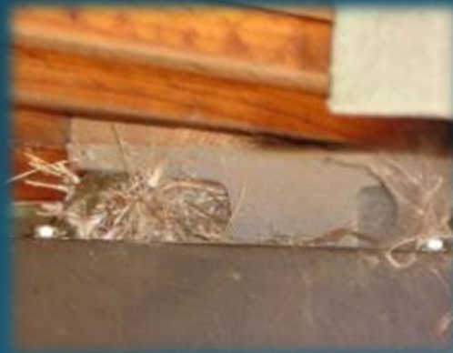
Rodent nest in crawl space
